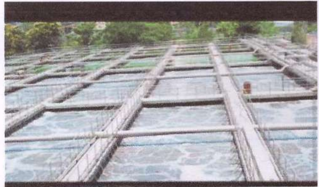
Air blower tank
